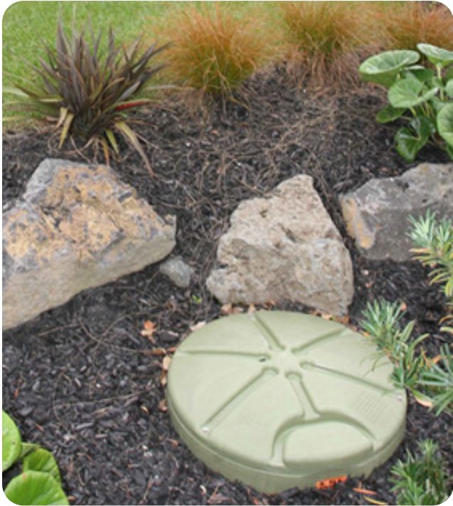
Pressure sewer lids are typically placed in a garden near the home.
